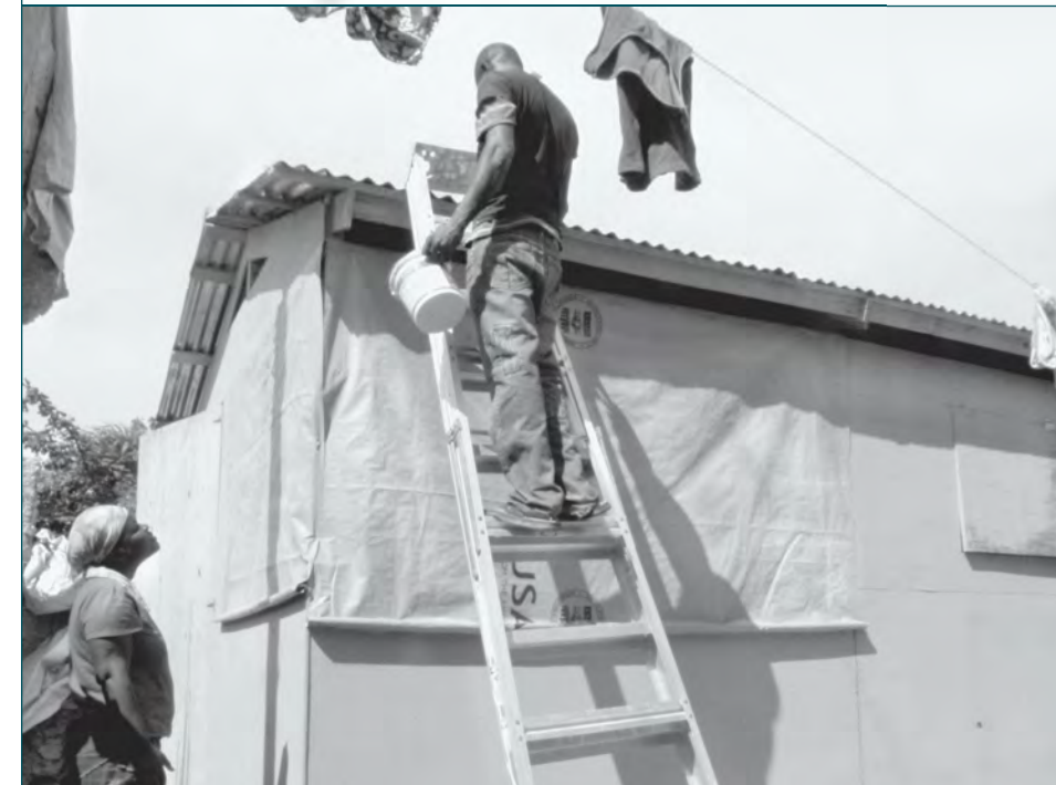
A Ti Shelter owner paints his new home in the Christ Roi neighborhood of Port-au-Prince.
