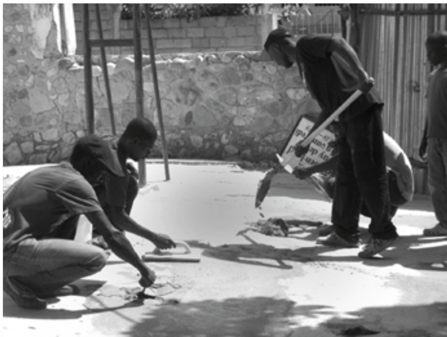
Students in the masonry class learn to fill, patch and smooth cracks in the concrete.
