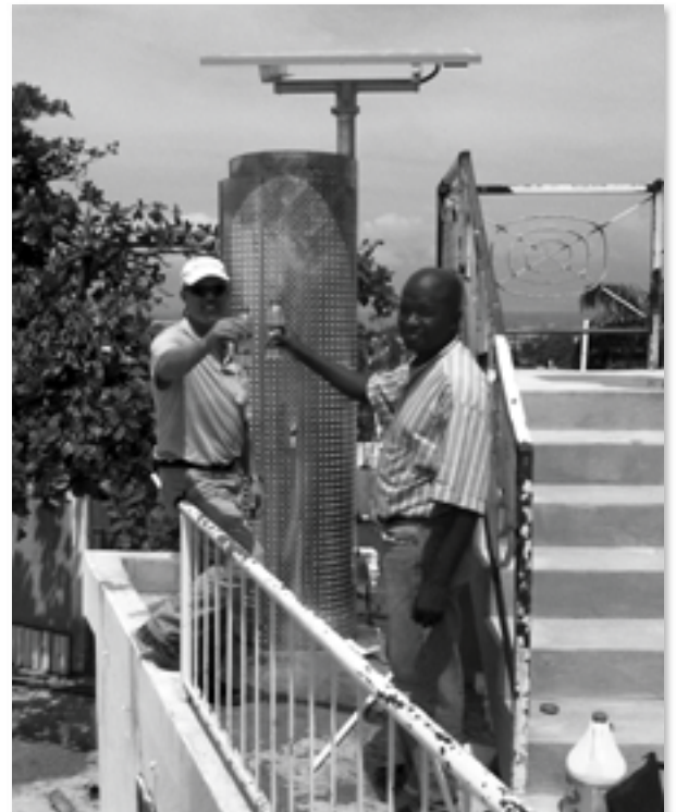
Jack Barker of Innovative Water Technologies and creator of the Sunspring system, and Executive Director Max Delices toast the installation of the water purification system at HSJ.
